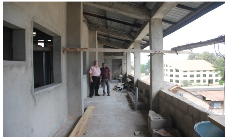
Bill standing with a student on the 2 nd floor that PAtHs will occupy of the new WAAST building.
